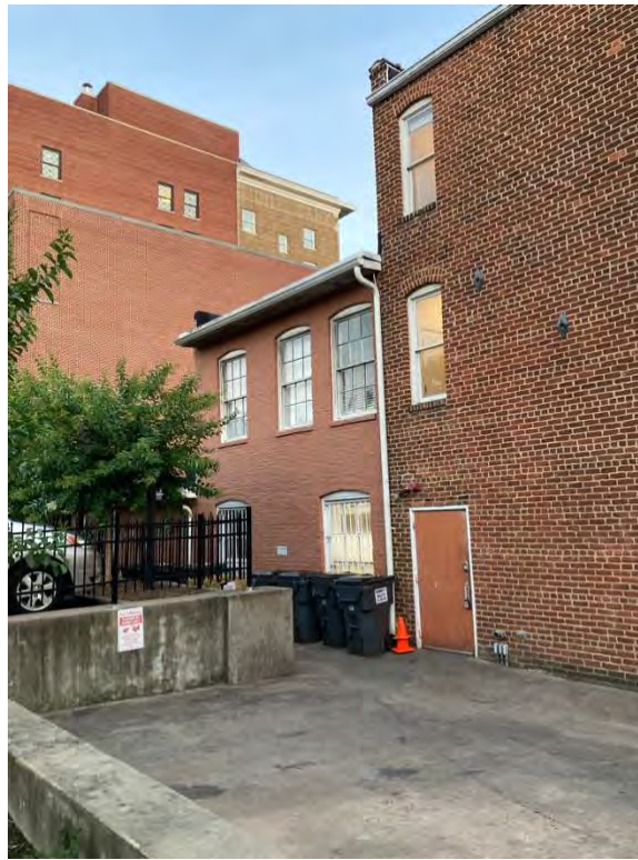
Figure 2: Oblique view towards rear of 105 East Main Street and window proposed for door conversion.
