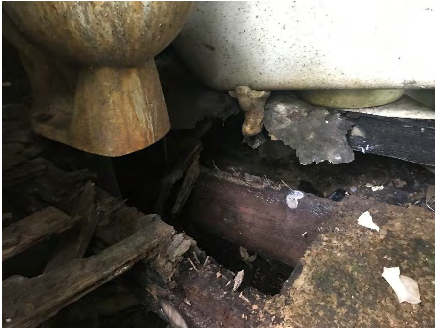
Interior detail – bathroom floor damage
