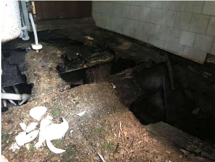
Interior detail – bathroom floor damage
