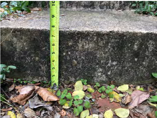
concrete steps - bottom riser is 7.5"
