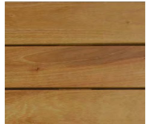
Black Locust Decking (multi-coat clear finish) at balcony floors and stair treads and landings
