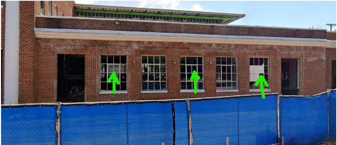
North façade – center west (Google street view). Openings where heaters are proposed.
