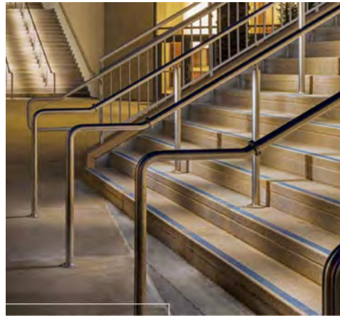
Handrail Precedent Anodized Aluminum Tube Rail Return to ground at top and bottom
