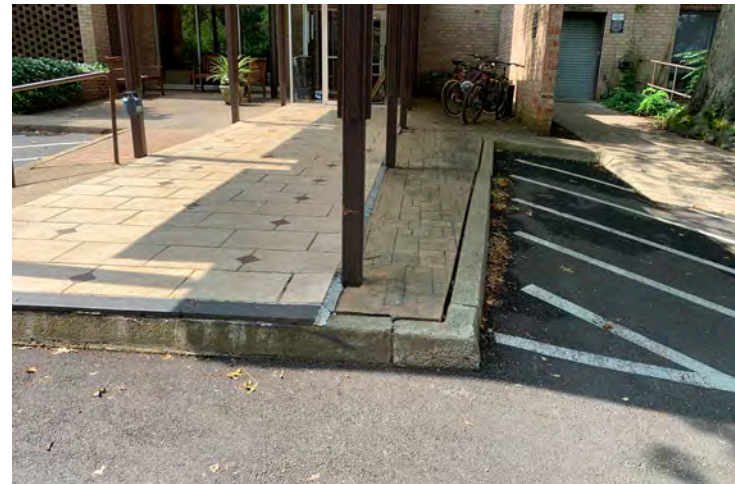
TOP SURFACE ELEVATION OF TILE AND ABUTTING PAVING DOES NOT MATCH
