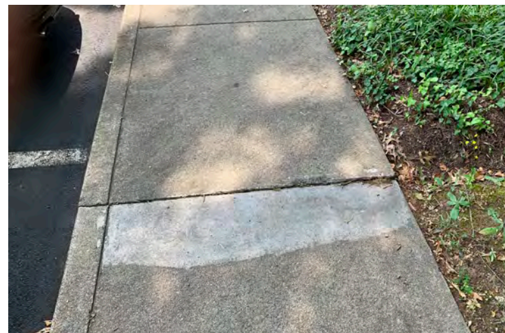
CHANGE IN LEVEL AT WALK JOINTS DOES NOT COMPLY WITH ADA REQUIREMENTS
