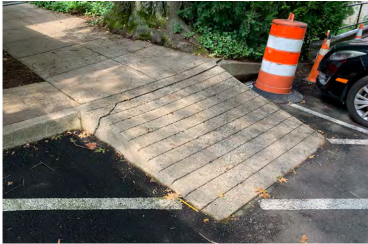
RAMP IS DANGEROUS TO NAVIGATE
