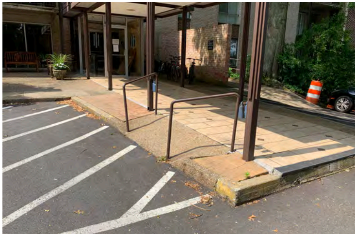
CURB RAMP IS NOT ADA-COMPLIANT
