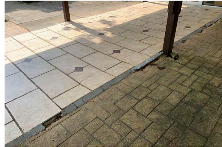
CERAMIC TILES ARE SLIP HAZARDS; TILES ARE LIFTING UP
