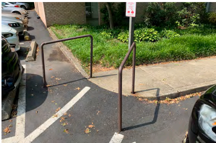
CURB RAMP IS NOT ADA-COMPLIANT
