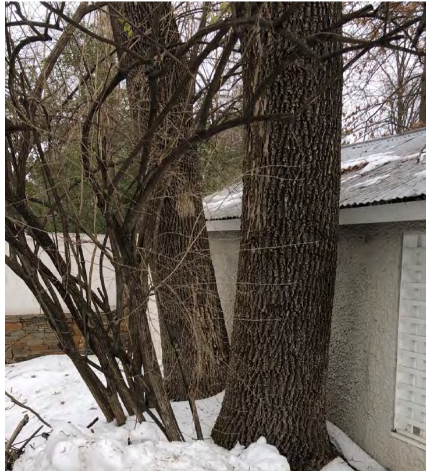
Base of ash trees growing into shed
