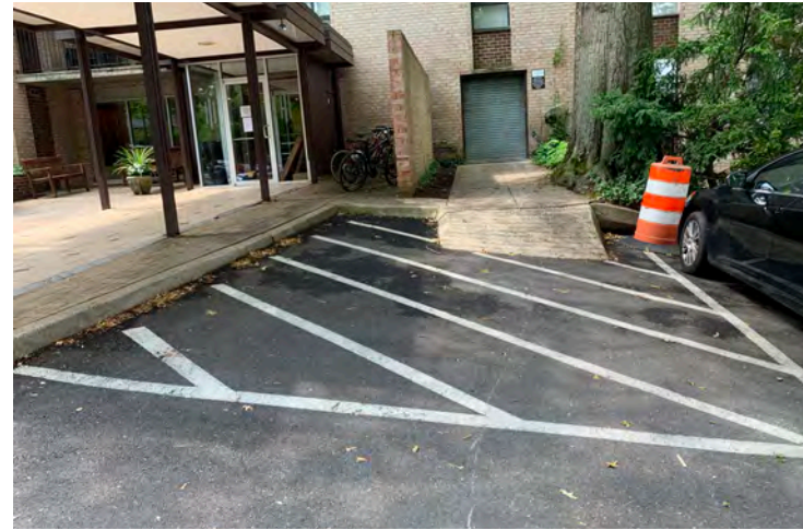
RAMP IS DANGEROUS TO NAVIGATE
