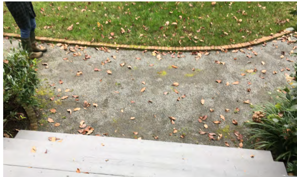
Crushed stone landing to be replaced with bluestone
