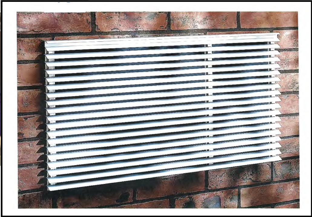
Thru-wall air conditioners on south and west elevations to be removed, masonry openings infilled and covered with Grainger architectural grilles. (Grilles will not function for ventilation, but as a decorative cover for the wall repair.)
