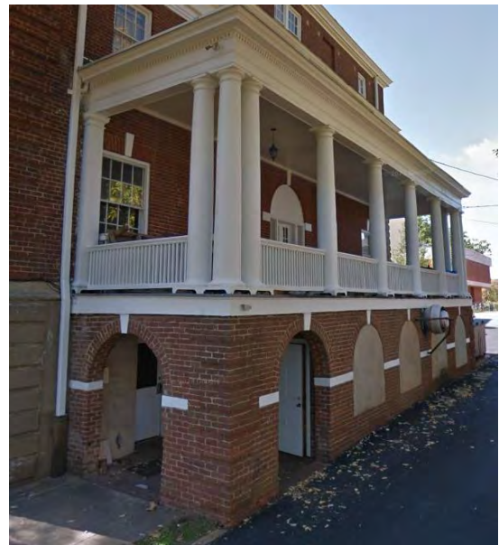
Figure 2: Filled-in arched basement openings at 165 Rugby Road
