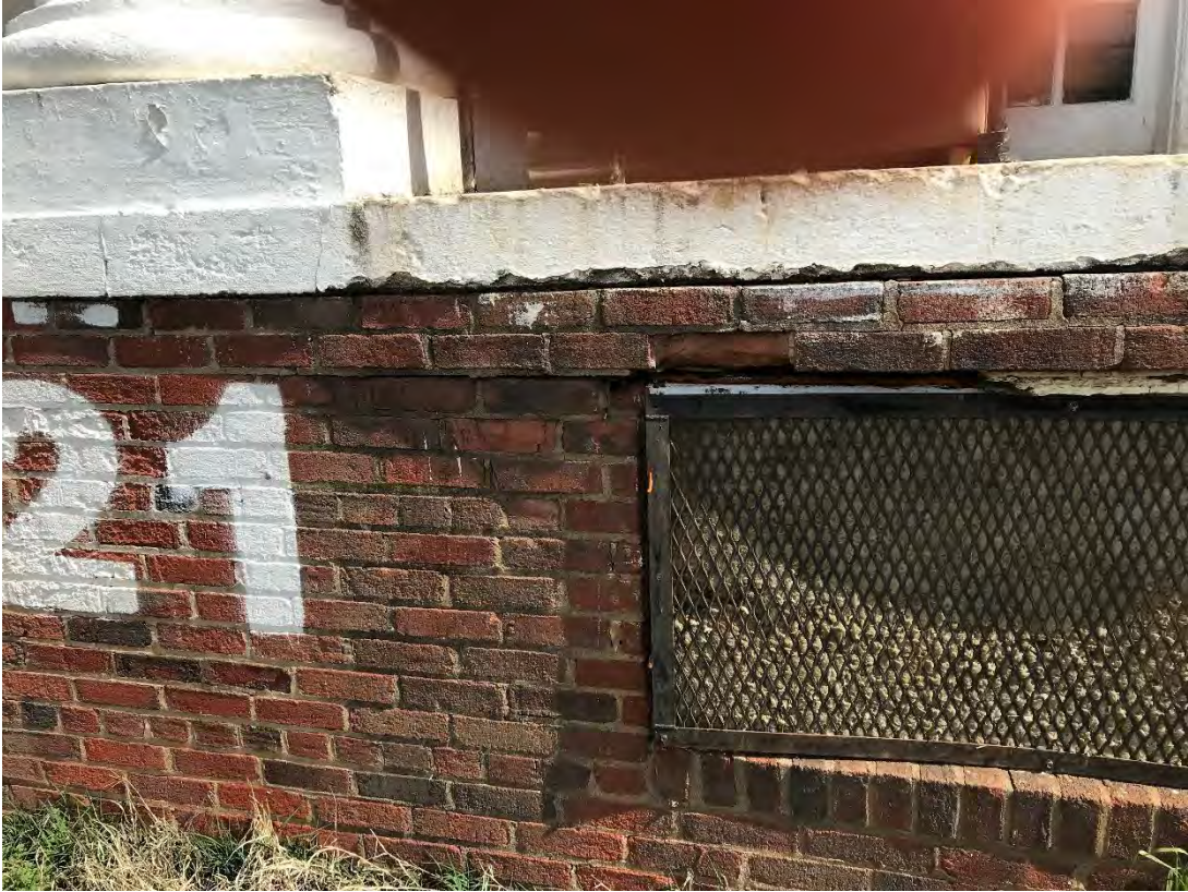
Detail photos of existing window conditions (windows covered-up by insulation and screens).
