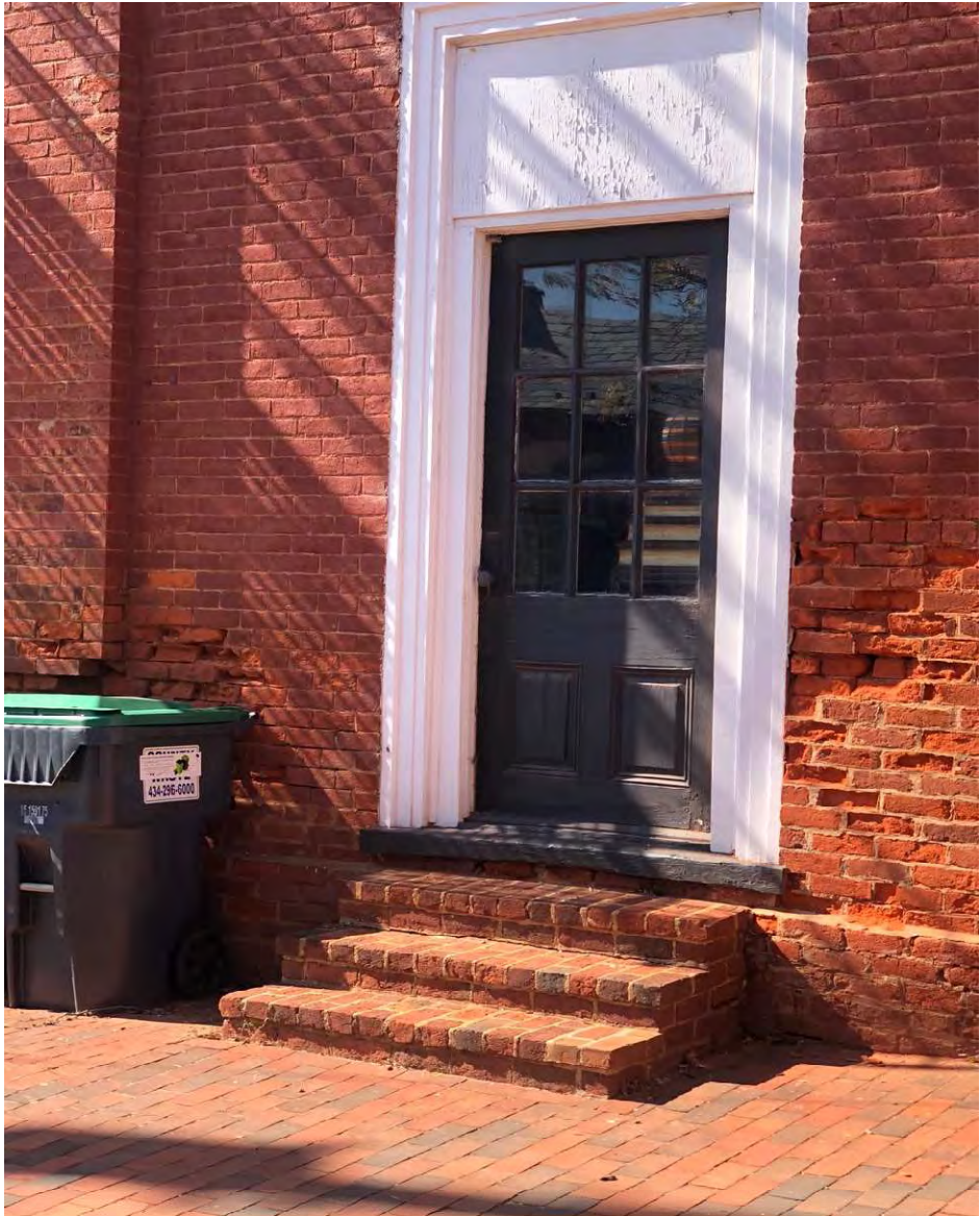
PHOTO 19 – REMOVE DOOR AND STEPS TO RIGHT OF PORTICO – REPLACE WITH ORIGINAL WINDOW
