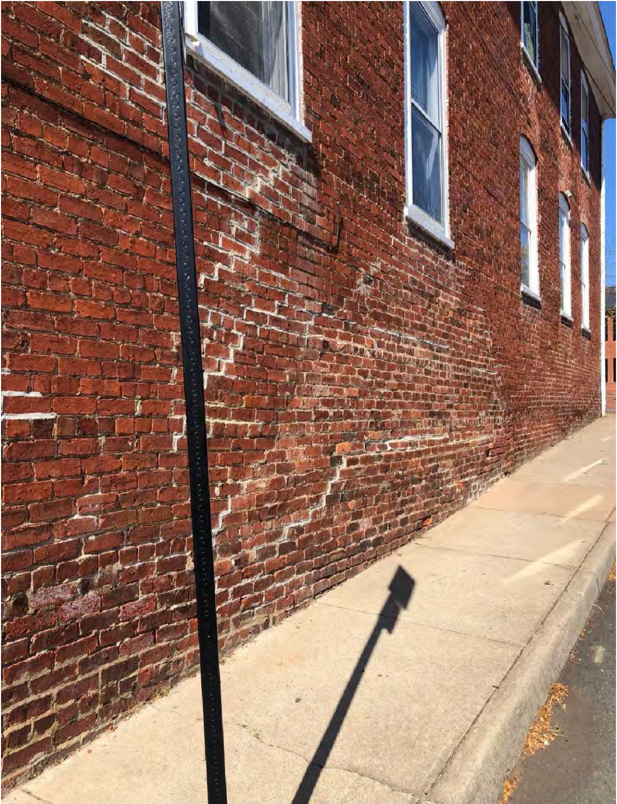
PHOTO 6 – MANY VARIATIONS OF MORTAR AND BRICKS – REPAIRS OVER THE YEARS
