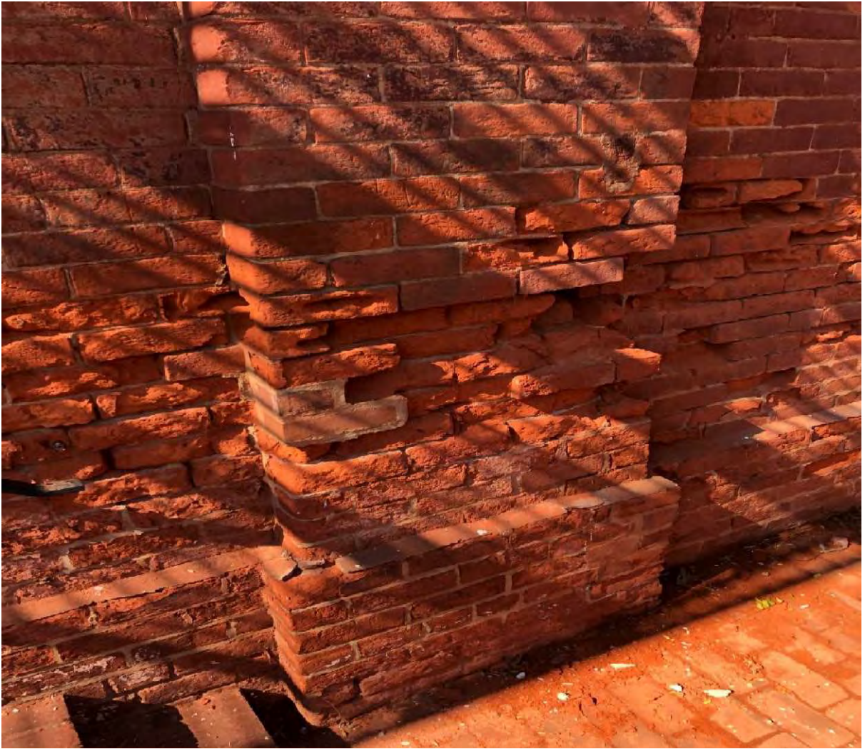
PHOTO 3 – FAILING BRICK CONDITION
