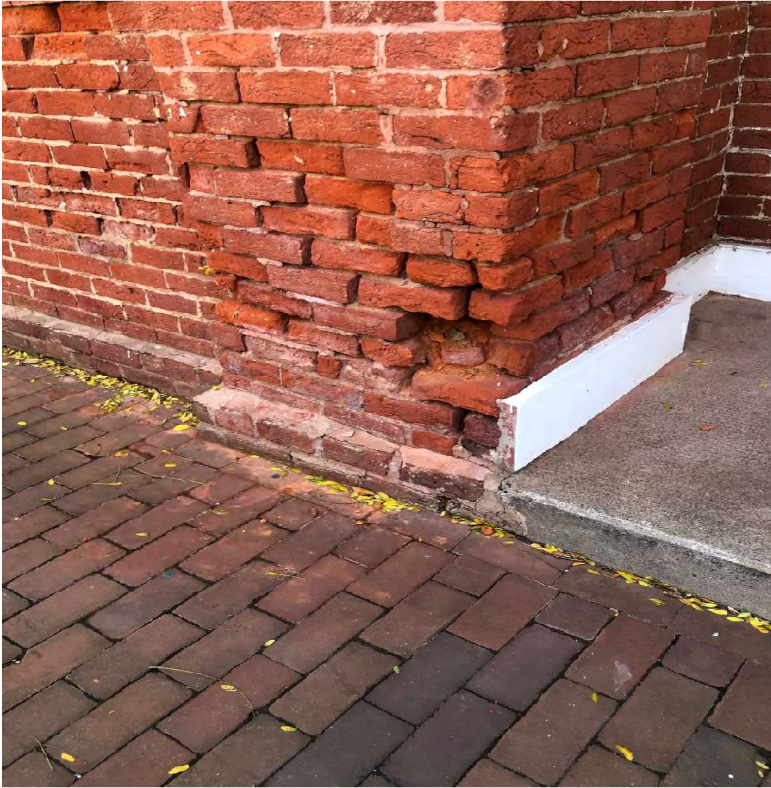
PHOTO 4 – FAILING BRICK CONDITION
