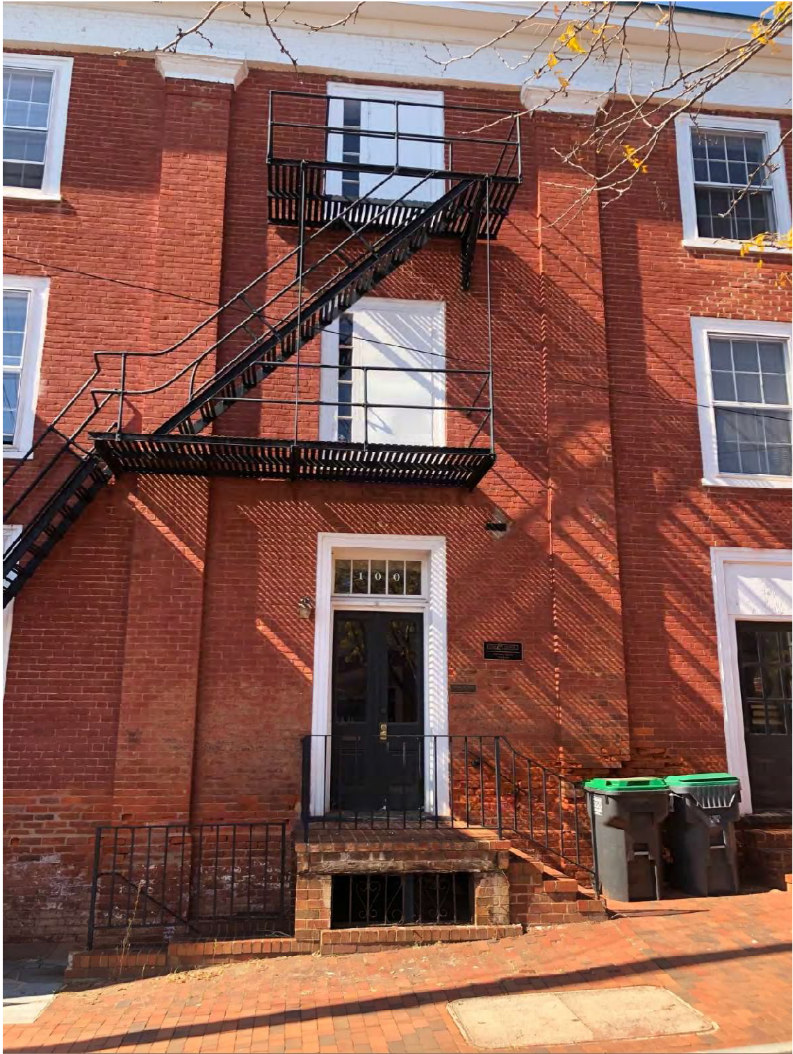
PHOTO 10 – FAILING BRICK AT STREET LEVEL, FIRE ESCAPE TO BE WRAPPED BY PORTICO
