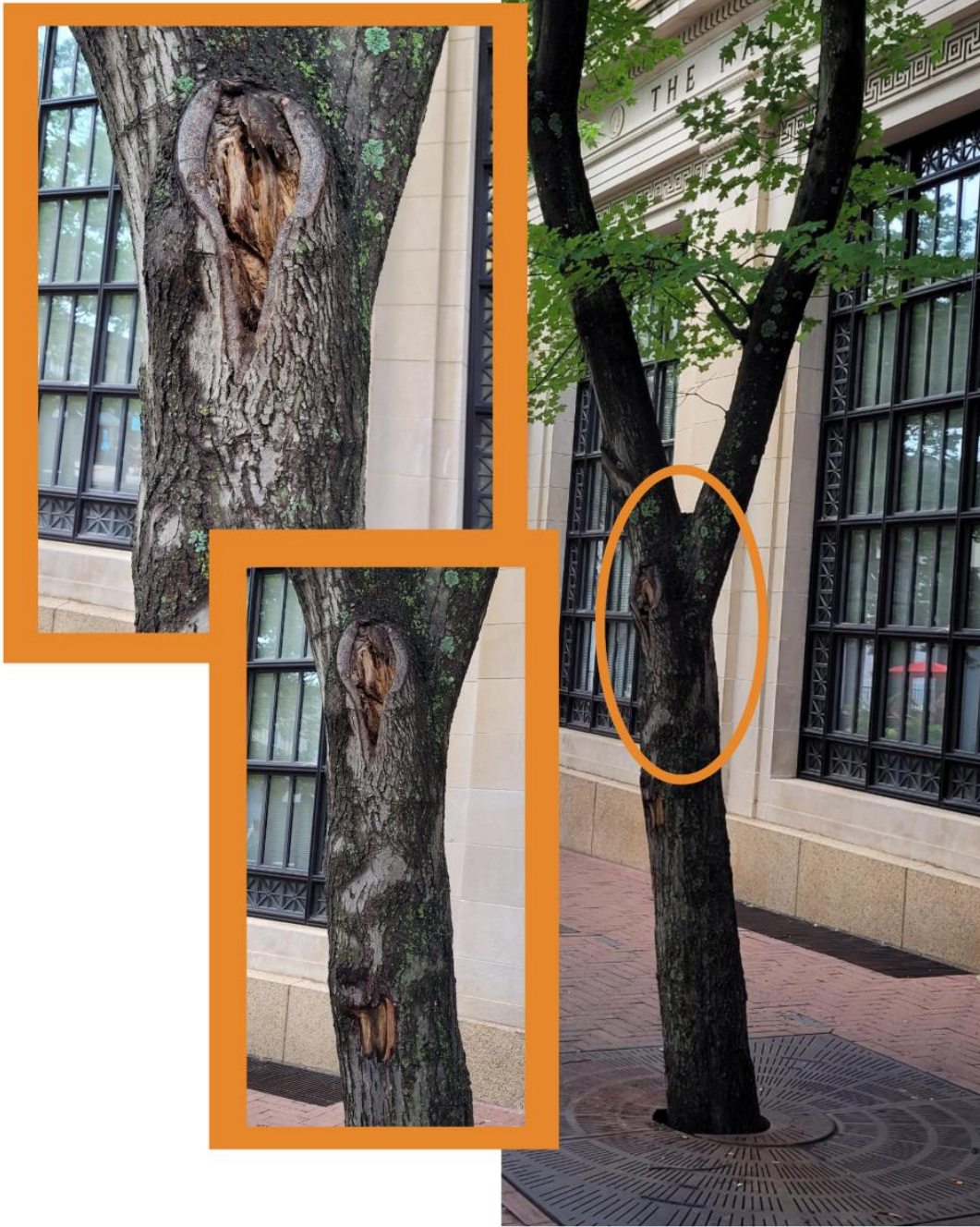
Figure 2: Red Maple, approximately 12 inches in diameter. Two significant wounds on tree bole (Approximately 4 feet high and 7 feet high respectively). Obvious internal decay at crotch, with additional infection evident in wilting leaves (probably Verticillium Wilt – unconfirmed currently). Location: Adjacent to Dining area – Petit Pois
