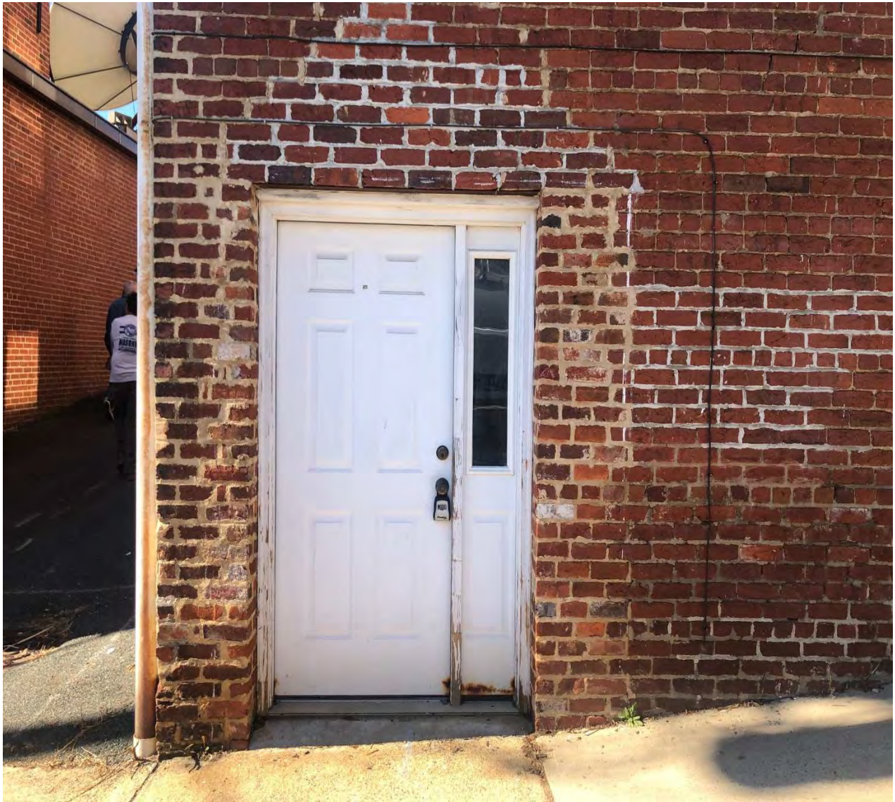
PHOTO 23 - EXISTING 6 TH STREET DOOR TO FUTURE GIFT STORE – TO BE REMOVED AND REPLACED WITH 15-LIGHT DOUBLE DOORS SHOWN BELOW
