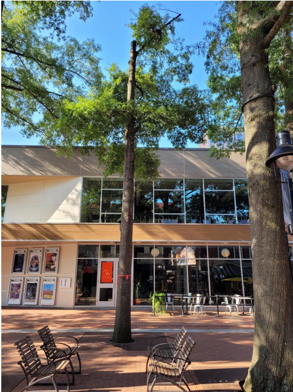
Figure 4: Willow Oak tree, approximately 12-14 inches in diameter. Tree displaying a few dead limbs in the upper canopy as well as large fruiting body on the stump (common indicator of severe internal decay). This tree has been heavily pruned over the years and is showing loss of vigor. Location: Across from Rockfish Brewing Company.
