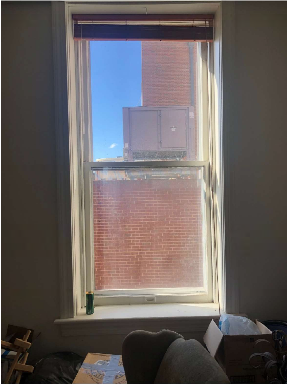
PHOTO 29 - VIEW OF AC CHILLER FROM "ANNEX ROOMS"
