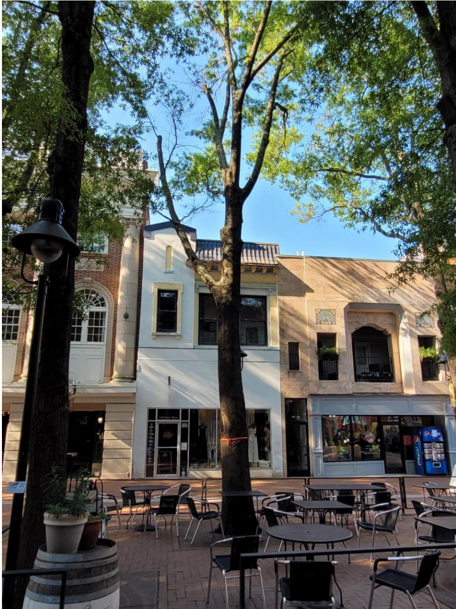
Figure 3: Willow Oak, approximately 22 inches in diameter. Obvious wound 5 feet high on tree bole, carpenter ant activity present. This wound is also flared and misshapen across the backside of the bole, further indicating instability. Location: Adjacent to 106 East Main Street
