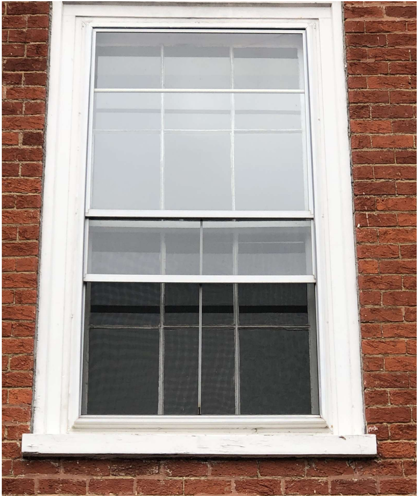
PHOTOS 1 -4 ORIGINAL WINDOW – NOTE MORTAR AT EDGES
