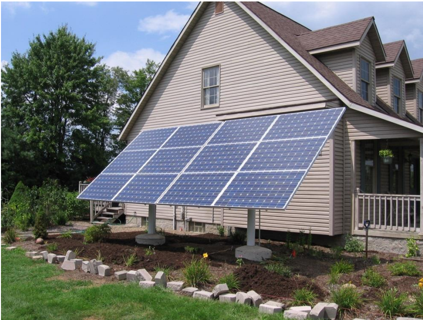
Ground-mounted solar energy systems in residential districts
