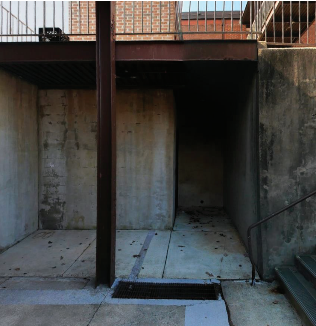
Unsafe and uninviting conditions
