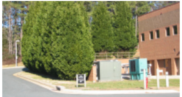
Large evergreen trees work with the grade of the site to obscure the view of utility equipment located behind this building.
