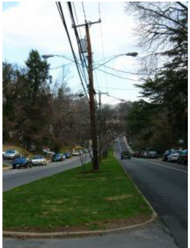
Above ground utilities visually dominate this green median on Jefferson Park Avenue.
