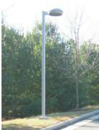
Full cutoff luminaires provide targeted lighting for commercial parking areas.
