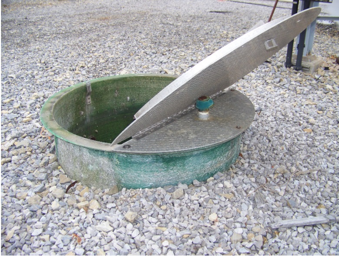
Figure 1: Wet Well Locking Manhole Lid
