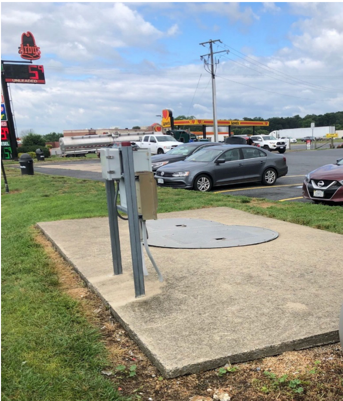
Figure 2: Pump Station Pad w. Unenclosed Control Panel
